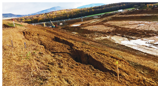
Fig. 4. Active landslides at 10.775–10.8 km (date: 25.10.2017).
