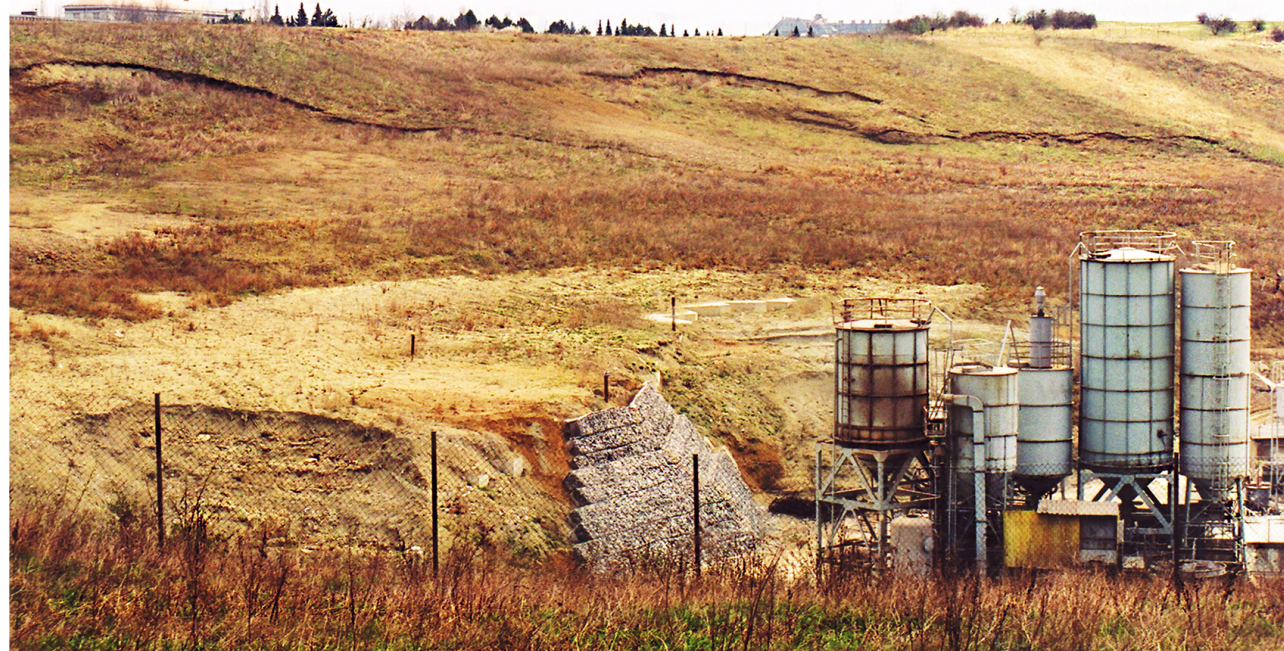
Fig. 9. Ponava, Cimburkova Street, landslide behind Tesco department store during its construction.
