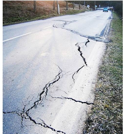
Fig. 13. Bystrc, Rakovecká Street, landslide reactivated in March 2016. Heavily damaged road.
